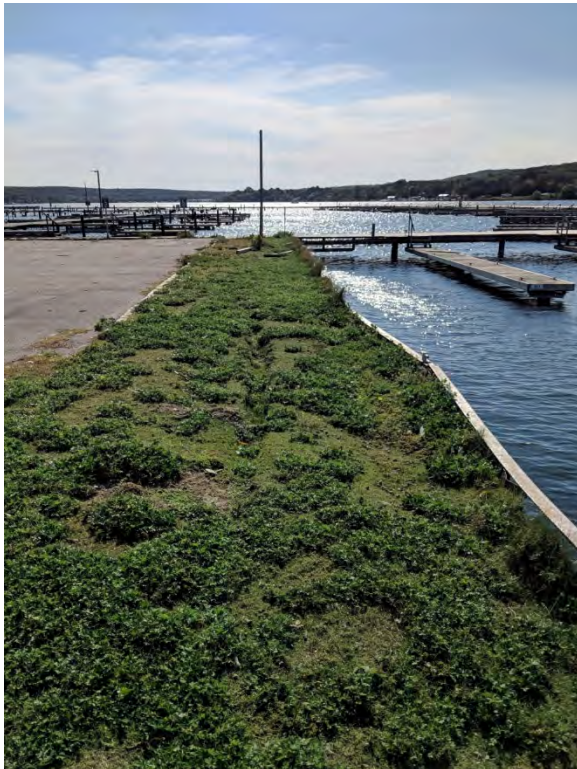
Photo 17 – Segment 7 - Failed Area
