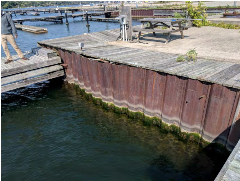
Photo 8 – Segment 2 – Failed Area
